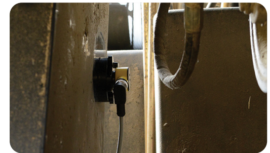
Back of elevator
